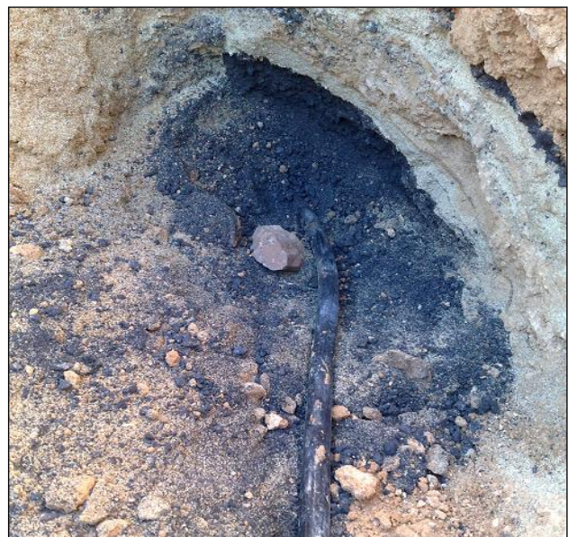
Fig. 9. Consumed anode ground bed in Brega CP system
