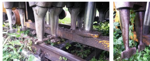
Fig. 7. a) Excessive consumption of the working surface of the hardfacing and the base material of the clamp and b) A clamp with correct technical parameters
