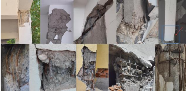
Fig. 4. Examples of damage to RC columns due to different reasons
