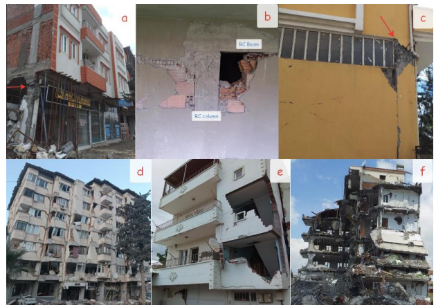
Fig. 3. Structural damages caused by different structural negativities a) pounding effect, b) strong beam-weak column, c) short column, d) irregularity in plan, e) heavy overhang, f) lack of RC frame
