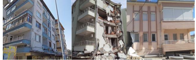
Fig. 2. Examples of damages caused by soft/weak story
