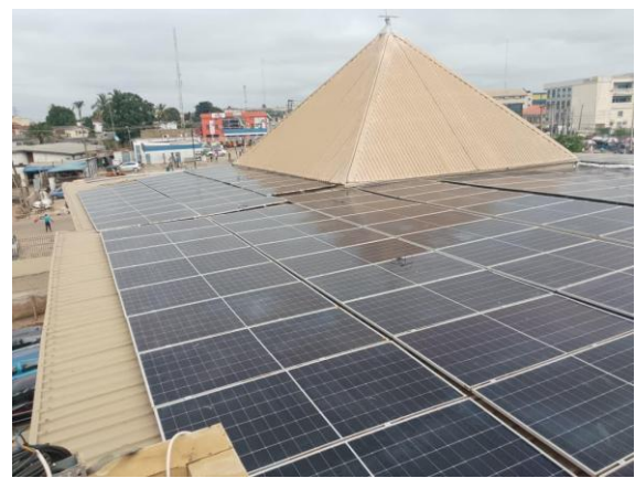
Fig. 2. The solar panels for the hybrid hydrogen-battery microgrid
